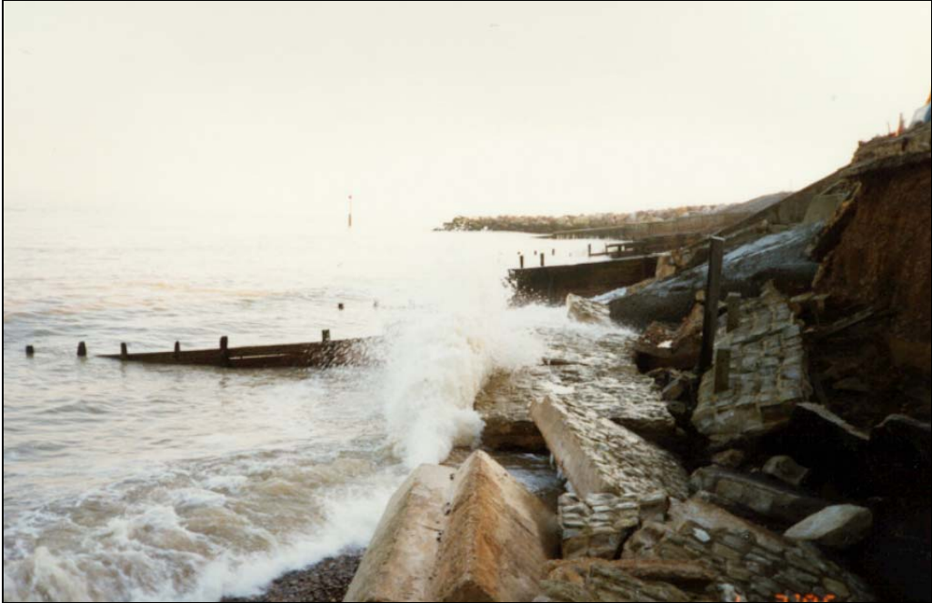
Figure 5.4 – Failed Seawall at Reculver caused by the 1996 Storm
