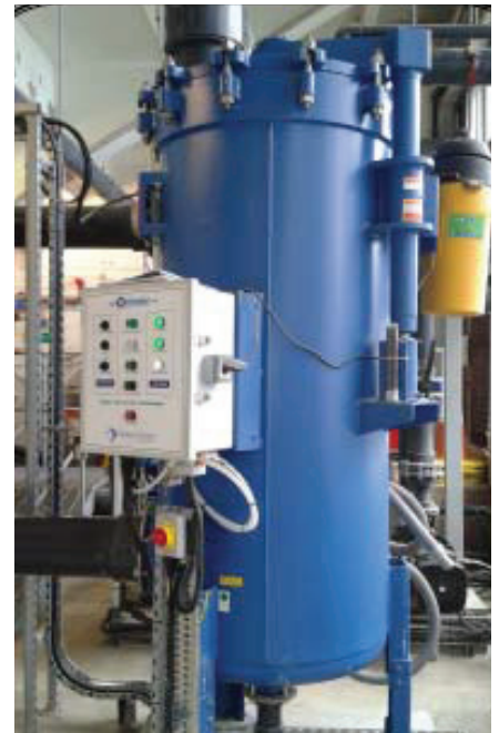
New water filter installed at Kingsmead Leisure Centre to improve water quality and save energy.
