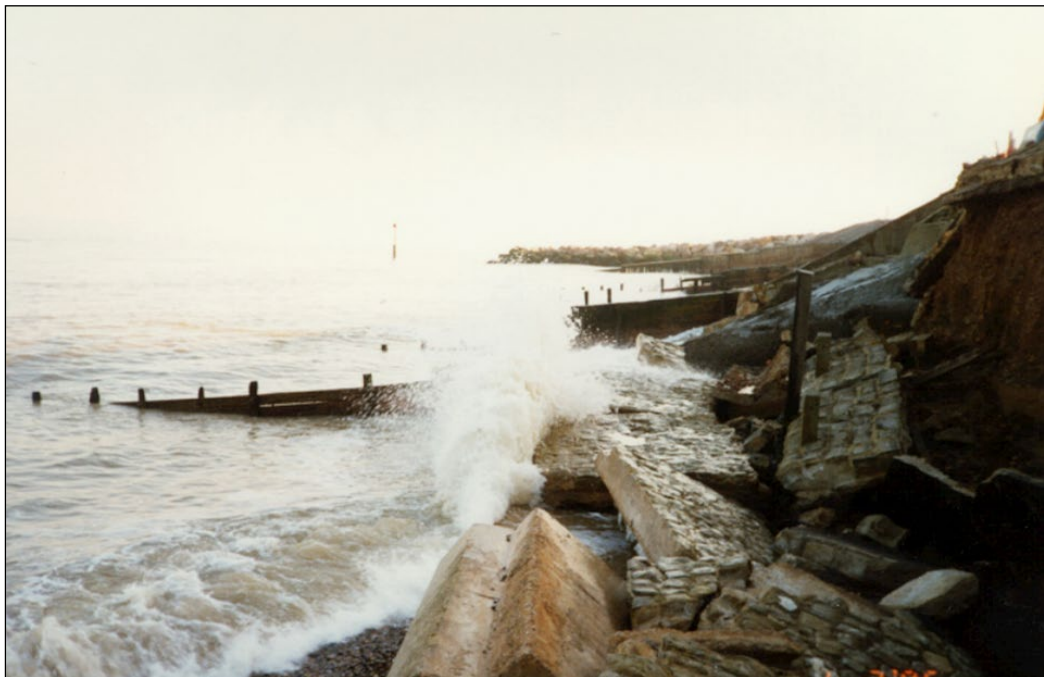
Figure 4.4 - Failed Seawall at Reculver caused by the 1996 Storm
