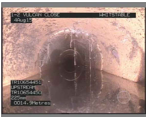
Photo: 006.JPG, VCR No.: 00004 14.9m, Fracture, circumferential, from 12 to 4 o'clock
