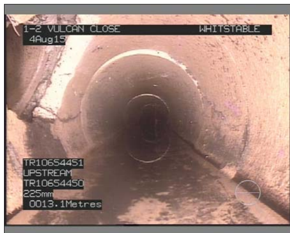
Photo: 005.JPG, VCR No.: 00004 13.1m, Connection defective, at 10 o'clock, 150mm diameter
