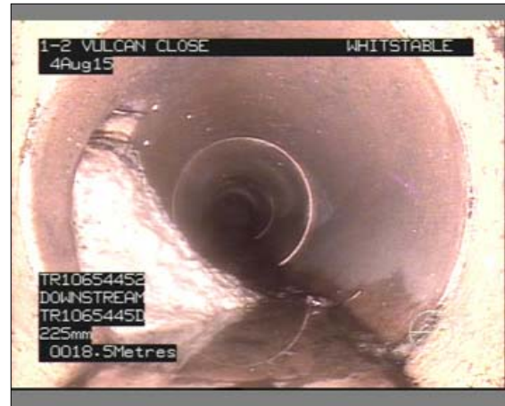
Photo: 009.jpg, VCR No.: 00005 18.5m, Encrustation, heavy, from 6 to 10 o'clock, 25% cross-sectional area loss
