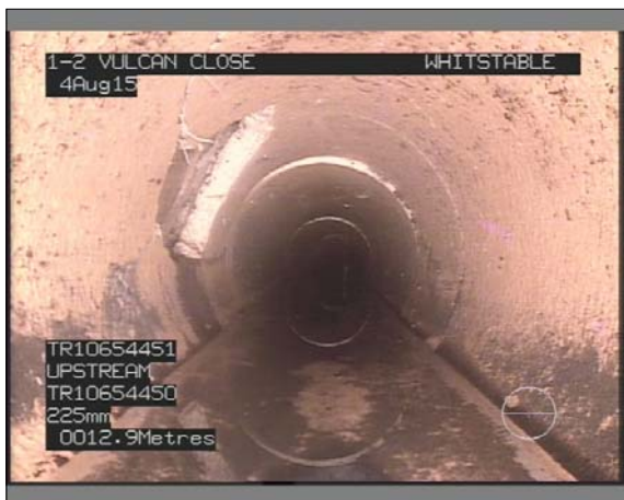
Photo: 004.JPG, VCR No.: 00004 12.9m, Cracks, multiple, from 12 to 12 o'clock
