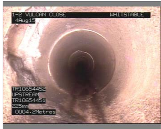
Photo: 003.jpg, VCR No.: 00003 4.3m, Connection, at 10 o'clock, 150mm diameter
