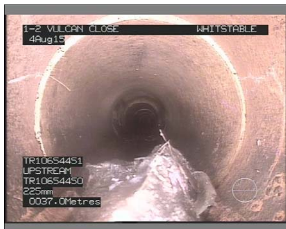
Photo: 007.JPG, VCR No.: 00004 37m, Fracture, longitudinal at joint, at 2 o'clock
