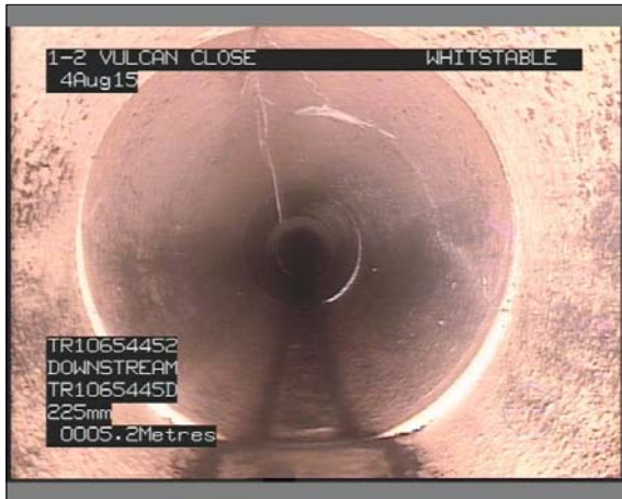
Photo: 008.JPG, VCR No.: 00005 5.2m, Crack, circumferential at joint, from 12 to 5 o'clock
