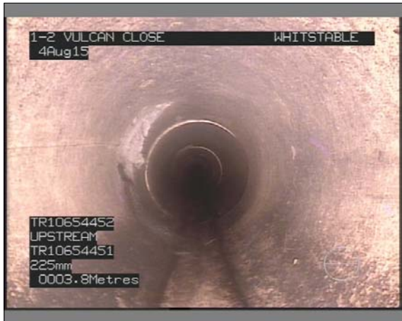
Photo: 002.JPG, VCR No.: 00003 3.8m, Crack, longitudinal, at 10 o'clock
