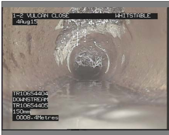
Photo: 001.JPG, VCR No.: 00002 8.4m, Hole in sewer, from 9 to 1 o'clock
