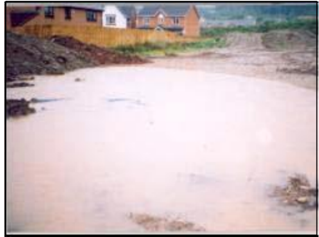
Excessive/unnecessary soil strip
