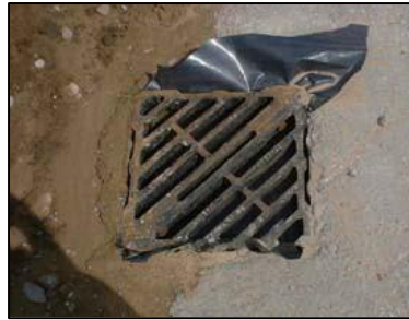
Protected Drain using Visqueen
