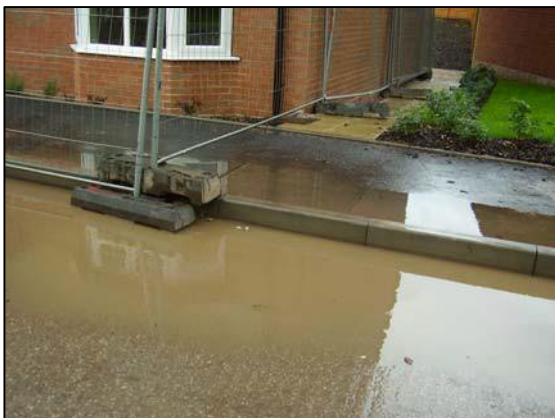
Terram not maintained leading to blockage and resulting in ponding of silty water
