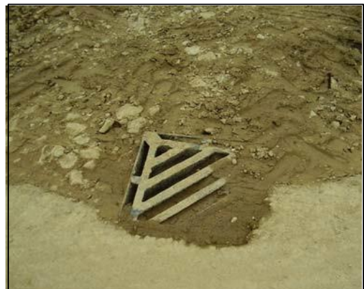
Gully unprotected allowing silt to block drain
