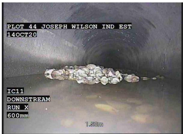
006.jpg, 00:00:14, 1.50 m Settled deposits, coarse, 30% cross-sectional area loss, start
