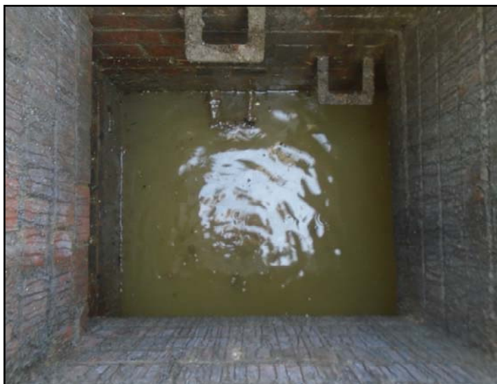
IC15 ASSUMED SURFACE WATER NO FOUL PRESENT AND SMELLS OILY
