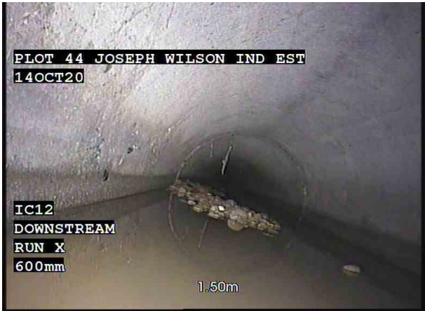
007.jpg, 00:00:13, 1.50 m Settled deposits, coarse, 30% cross-sectional area loss, start
