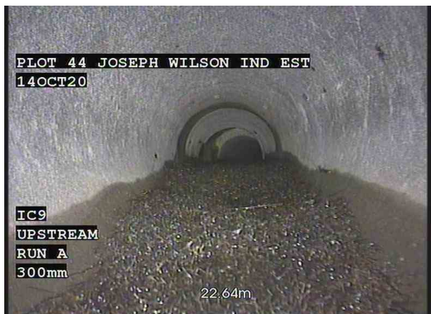
005.jpg, 00:02:08, 22.64 m Roots, mass, 30% cross-sectional area loss
