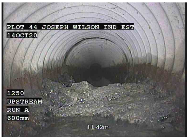
010.jpg, 00:01:35, 11.42 m Settled deposits, coarse, 35% cross-sectional area loss
