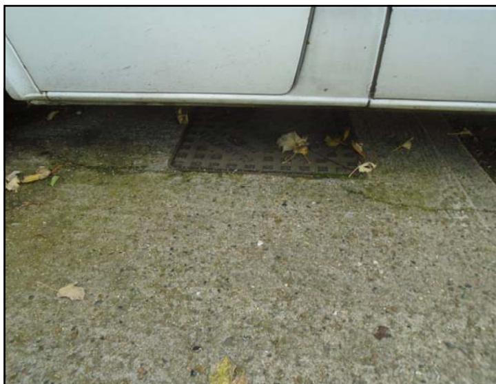
IC16 UNABLE TO LIFT ASSUMED TO BE ON SURFACE WATER SYSTEM
