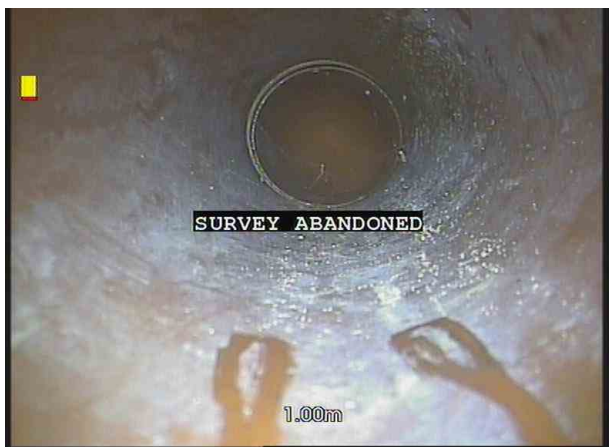
003.jpg, 00:01:09, 1.00 m Survey abandoned, Unable to continue round bends - assumm to blocked road gully
