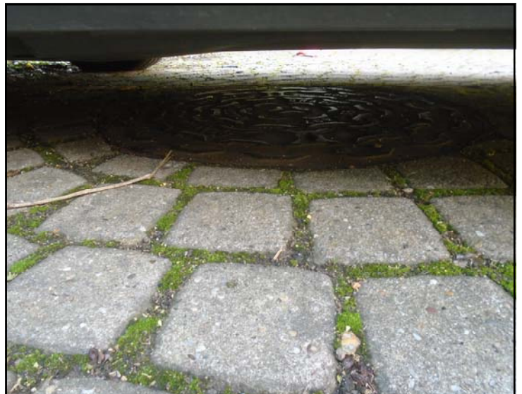
LOCATION OF IC10 OBSTRUCTED UNABLE TO LIFT UNDER CAR
