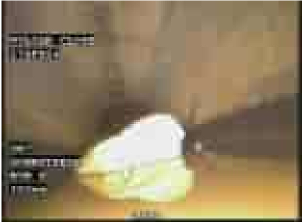
1, 00:00:23, 4.08 m Settled deposits, hard or compacted, 5% cross-sectional area loss
