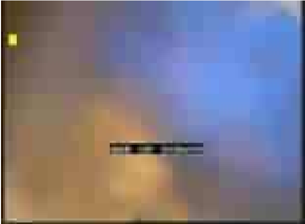
1, 00:01:04, 9.15 m Finish node, gully, reference: SW16-A, At assumed gully - debris filled
