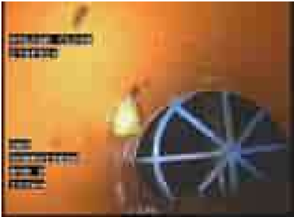
1, 00:00:14, 0.53 m Settled deposits, hard or compacted, 10% cross-sectional area loss
