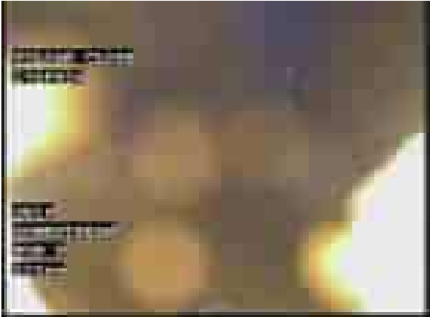
1, 00:00:20, 3.45 m Settled deposits, hard or compacted, 5% cross-sectional area loss, start
