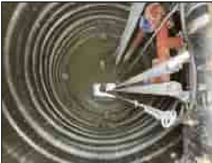
P.S.1. PUMP STATION
