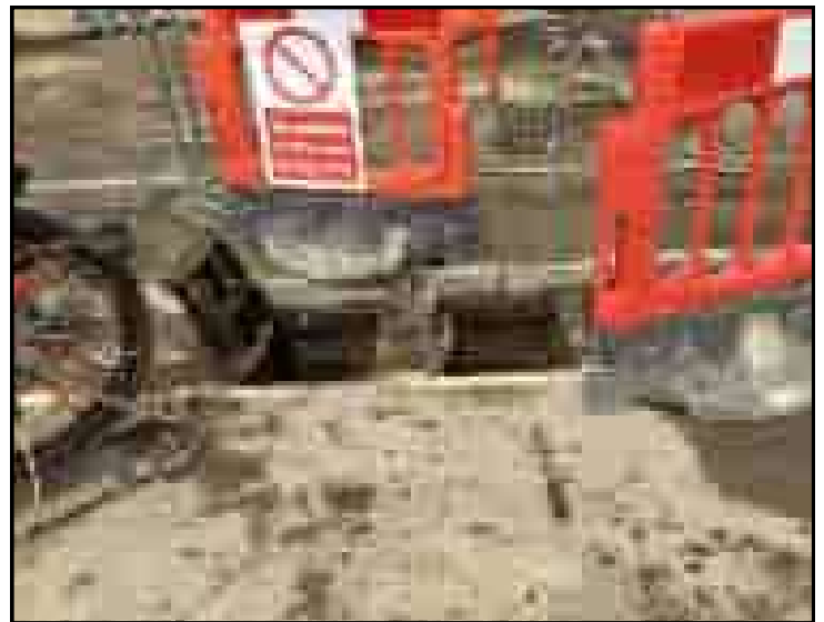
LOCATION OF GULLY 1 (LEFT OF PHOTO)
