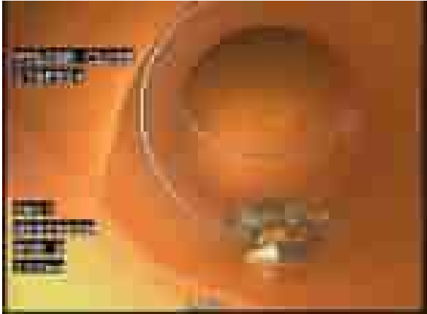
1, 00:00:37, 7.14 m Settled deposits, fine, 5% cross-sectional area loss
