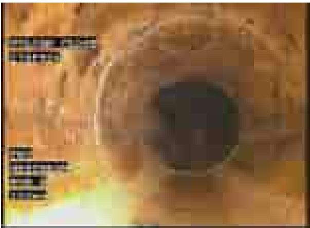
3, 00:01:09, 4.13 m Crack, circumferential from 07 o'clock to 11 o'clock
