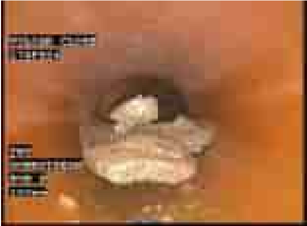
1, 00:00:33, 3.43 m Settled deposits, hard or compacted, 50% cross-sectional area loss
