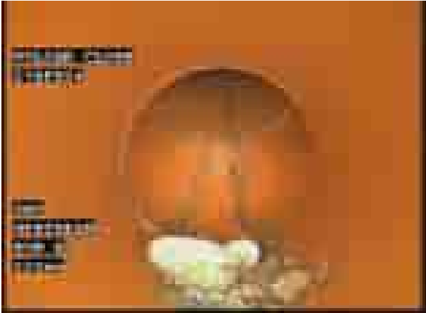
1, 00:01:11, 8.41 m Settled deposits, hard or compacted, 5% cross-sectional area loss
