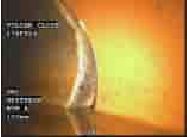
1, 00:00:20, 0.28 m Joint displaced, medium
