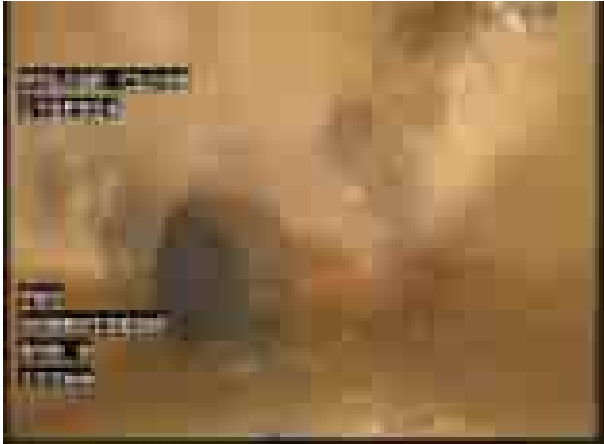
1, 00:00:44, 5.49 m Settled deposits, hard or compacted, 5% cross-sectional area loss
