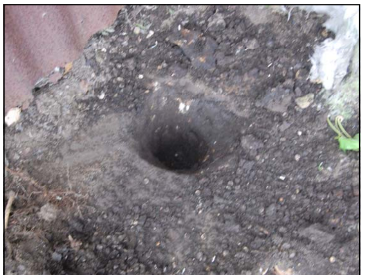
RWP 1, POSSIBLE GULLY / OUTFALL. UNABLE TO CCTV
