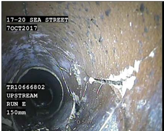
Photo: 022.jpg, VCR No.: 00009 0.5m, Crack, longitudinal, at 3 o'clock
