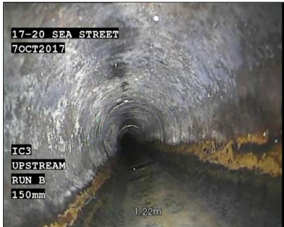
Photo: 018.jpg, VCR No.: 00007 1.22m, Encrustation, light, from 4 to 8 o'clock, Start
