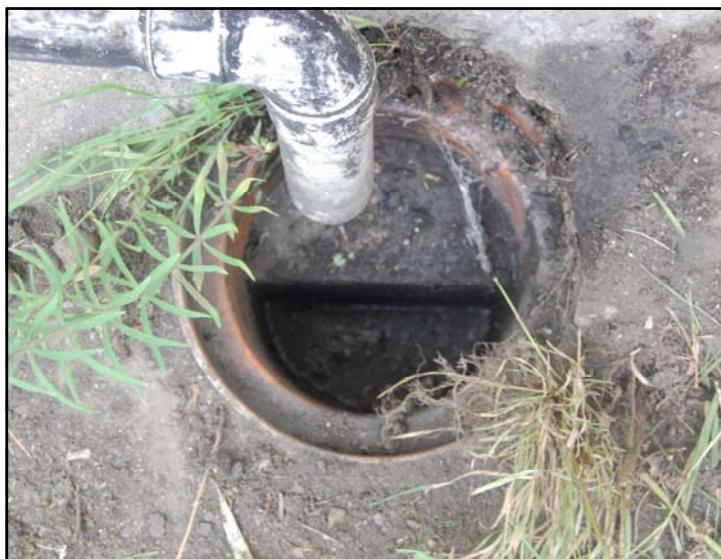
FOUL GULLY 1 - UNABLE TO CCTV
