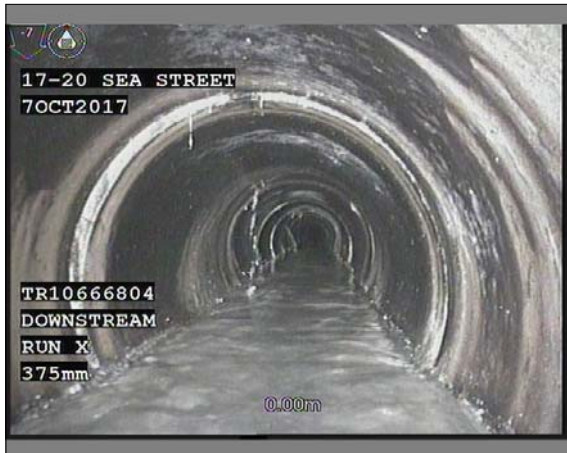
Photo: 003.JPG, VCR No.: 00002 0m, Debris, 10% cross-sectional area loss, Start
