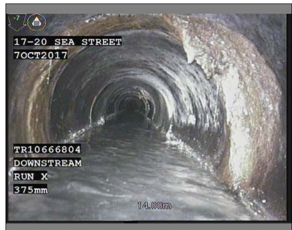
Photo: 010.JPG, VCR No.: 00002 14.88m, Encrustation, medium at joint, from 12 to 4 o'clock, 10% cross-sectional area loss
