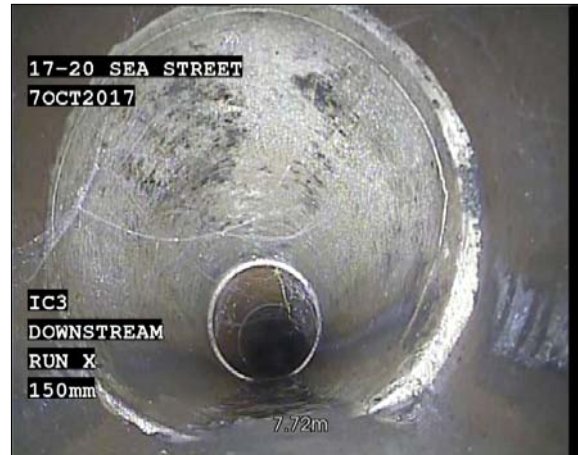
Photo: 021.jpg, VCR No.: 00008 7.72m, Crack, circumferential at joint, from 9 to 3 o'clock
