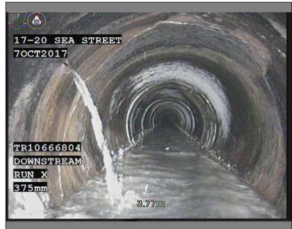
Photo: 008.JPG, VCR No.: 00002 3.77m, Infiltration, runner at joint, from 10 to 11 o'clock
