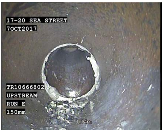
Photo: 024.jpg, VCR No.: 00009 1.14m, Debris, 5% cross-sectional area loss, Start
