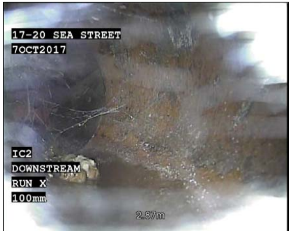
Photo: 017.jpg, VCR No.: 00006 2.87m, Debris, 5% cross-sectional area loss, Start
