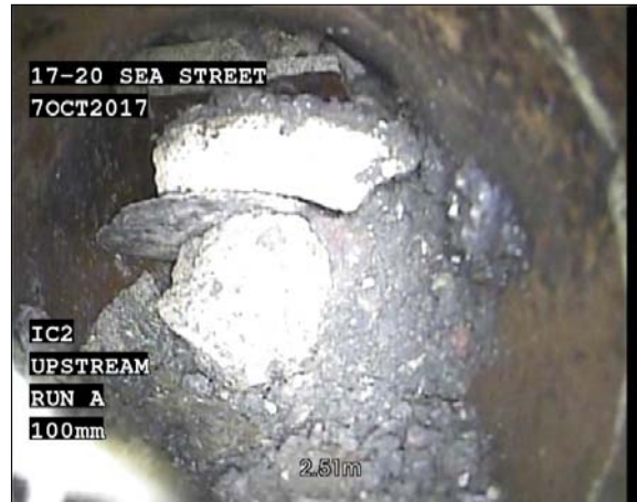
Photo: 013.jpg, VCR No.: 00003 2.51m, Debris, 95% cross-sectional area loss
