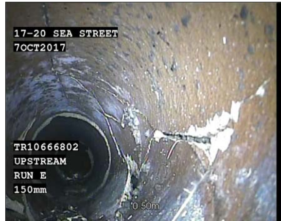
Photo: 023.jpg, VCR No.: 00009 0.5m, Hole in sewer, from 3 to 4 o'clock
