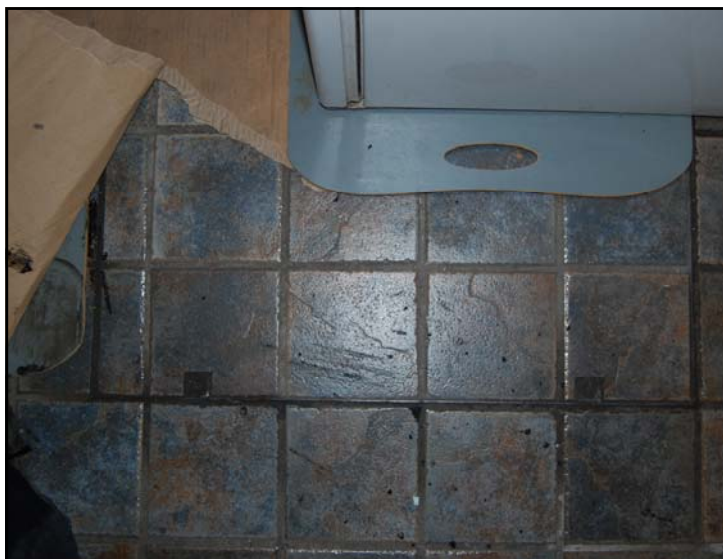
IC1 - UNABLE TO LIFT, OBSTRUCTED
