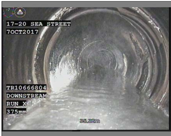
Photo: 011.JPG, VCR No.: 00002 35.32m, Infiltration, dripper at joint, from 10 to 9 o'clock
