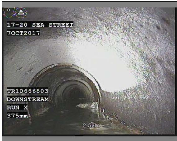
Photo: 001.JPG, VCR No.: 00001 2.52m, Debris, 10% cross-sectional area loss, Start
