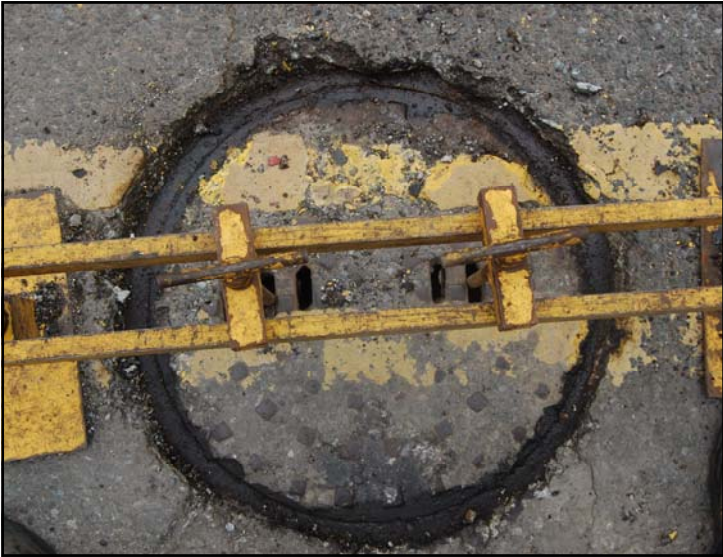
TR10666804. UNABLE TO LIFT, COVER SIEZED IN FRAME
