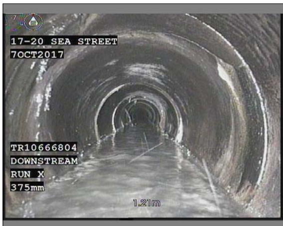
Photo: 005.JPG, VCR No.: 00002 1.21m, Fracture, circumferential at joint, from 12 to 2 o'clock
