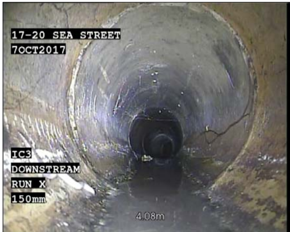
Photo: 020.jpg, VCR No.: 00008 4.08m, Roots, fine at joint
