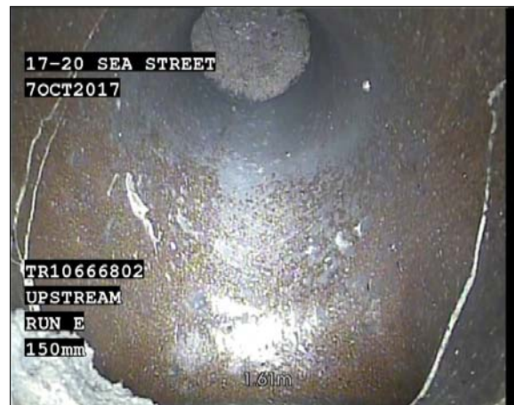
Photo: 025.jpg, VCR No.: 00009 1.61m, Crack, circumferential, from 3 to 10 o'clock
