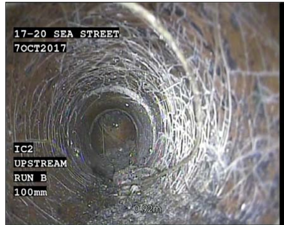
Photo: 015.jpg, VCR No.: 00004 0.92m, Debris, 5% cross-sectional area loss, Start
