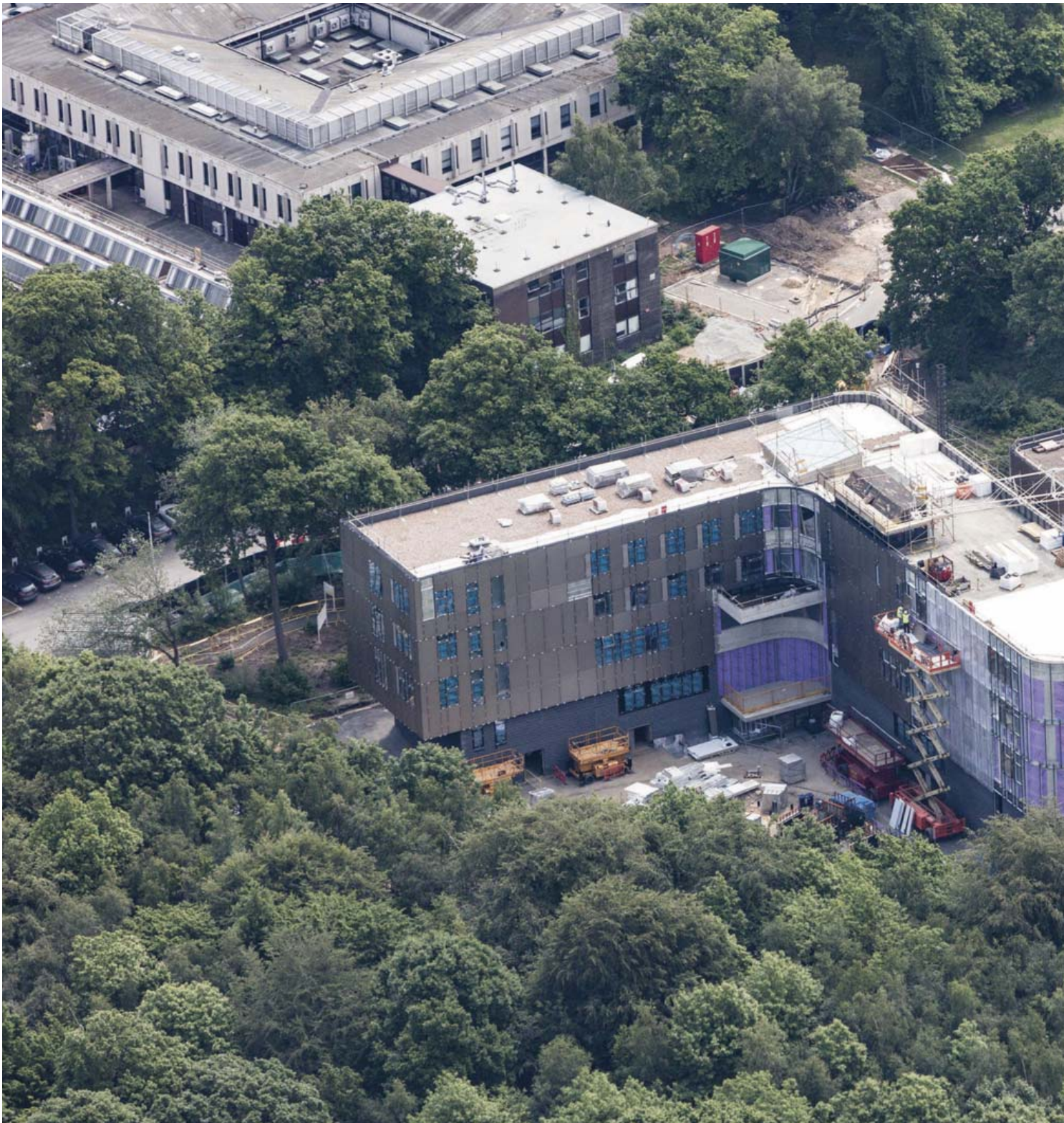
Figure 99: The Sibson Building in Brotherhood Wood nearing completion in 2017. Brotherhood Square is gradually taking shape in the top of the photograph
