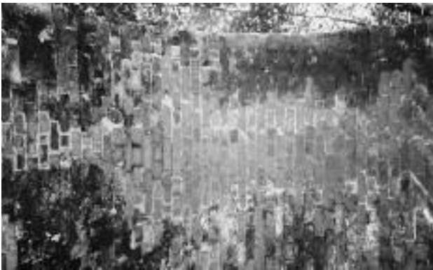
Detail of damaged brickwork at tunnel entrance
