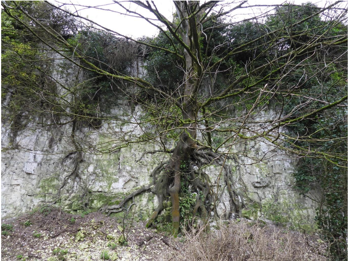
Figure 6 Tree growing out of chalk cliff face in Cooper's Pit
