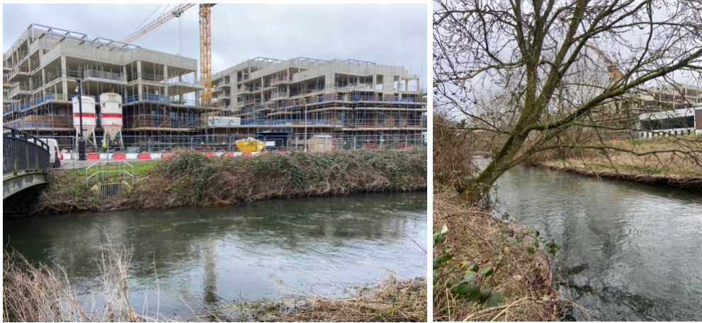
Figure 5.1 Great Stour Kingmead Riverside construction eroding river bank
