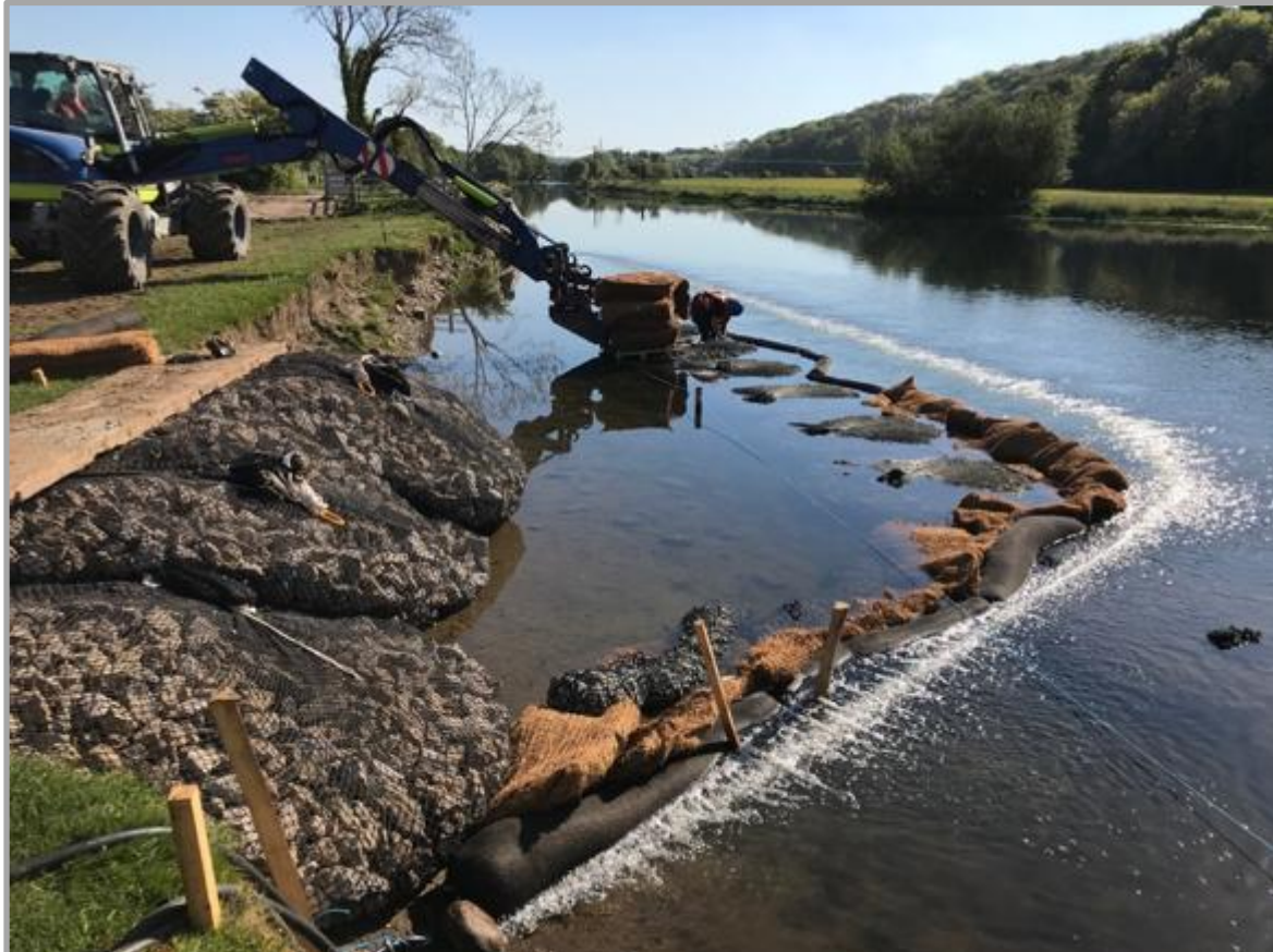
Figure 3-1 Silt Wattles, Silt Mats and Bubble Barrier to control sediment release (Photo courtesy of Frog Environmental).
